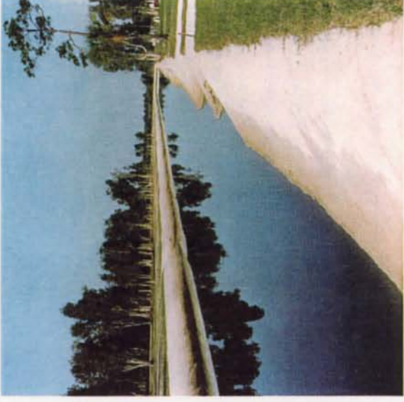
CLOSE VIEW OF SLOPING CONCRETE WALL No concrete caps to mar the canal beauty. Easy lawn mowing with no hand trimming.
